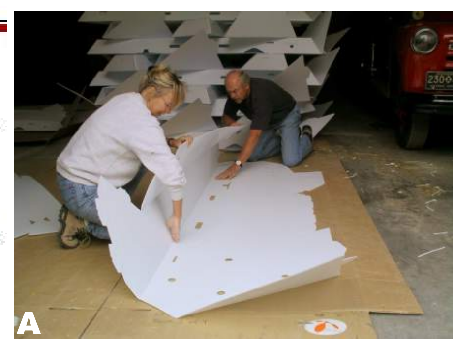
A Campground staff members, and our own on site "Icopod Techs," Terry and Pam Morrow, begin the construction. Shown here "exercising the seams in the pre-cut plastic sheets as they bend and fold the main support pieces that make up 90% of the Icopod. Behind them you can see complete pieces that have already been "exercised" and folded into place. These straight pieces will be joined together by the hooks and flaps to become the series of geometric triangles that you can see make up the unit. Ingenious engineering of the Icopod means that after assembly there are virtually no waste materials left over.
